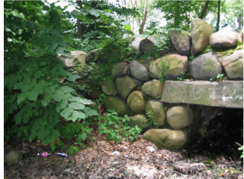
Photo 267 Bushes and plants growing from cracks on the south side of the east cheek wall; note the deeply eroded mortar joints.
