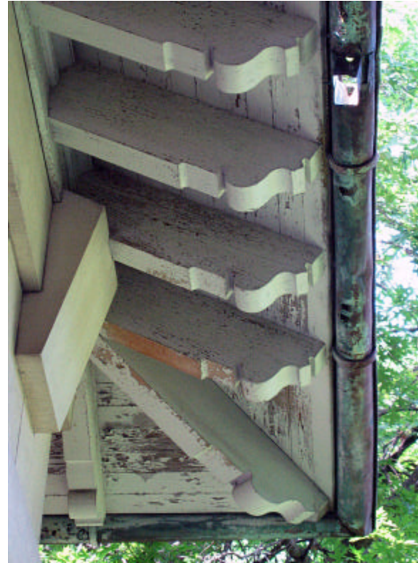
Photo 235 Carved ends of the wooden rafters and the beaded wood board sheathing; note the chipping and cracking of the paint on the rafters as well as the rotted wood sheathing. Also note the condition of the copper gutters and missing downspout.
