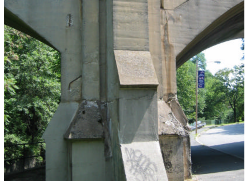
Photo 322 The base of this pier is severely damaged; note the exposed and rusting steel reinforcing in many locations.
