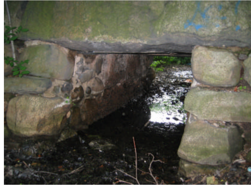
Photo 263 The box culvert under the bridge; note that some remedial patching with concrete and fieldstones is apparent.
