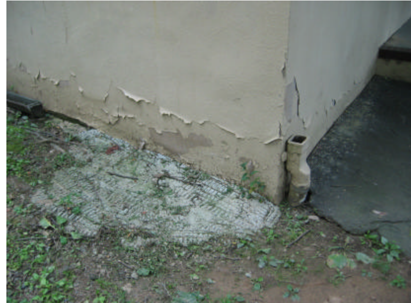
Photo 290 The base of the north wall showing cracked and peeling paint caused by water damage from a missing downspout; note the leftover concrete on the ground.
