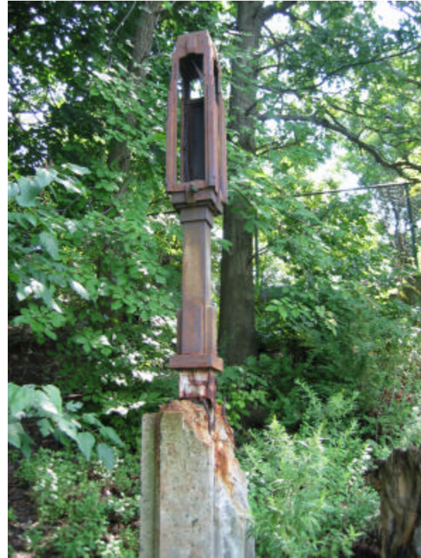
Photo 301 This lantern is covered with rust, and the concrete base has severely deteriorated; note the exposed and rusting steel reinforcing.
