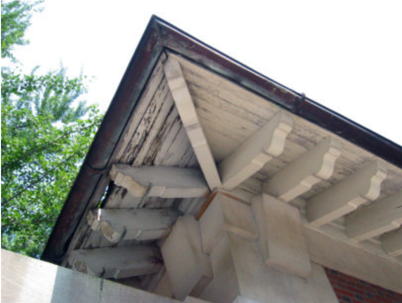
Photo 238 Copper gutters on the edges of each pavilion; note the poor condition of the eaves.
