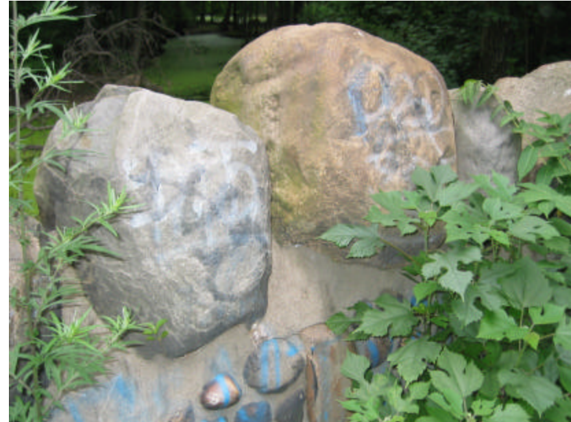
Photo 188 Detail of copingstones and mortar joints on the north cheek wall; note the graffiti and plant growth.
