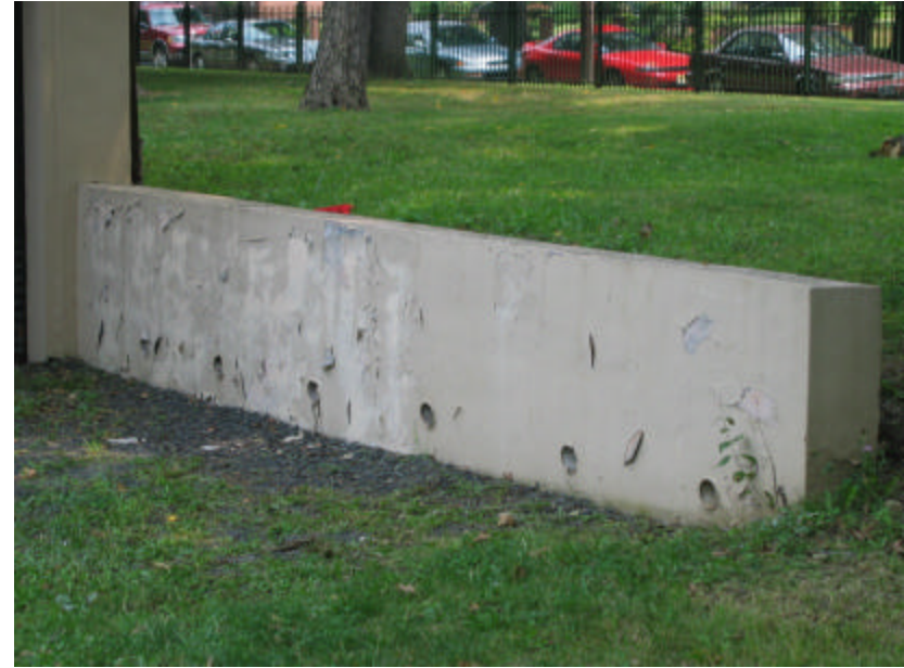
Photo 288 The concrete retaining wall has been damaged by water penetrating from the surrounding grade and freeze-thaw cycles; note the cracked and peeling paint.
