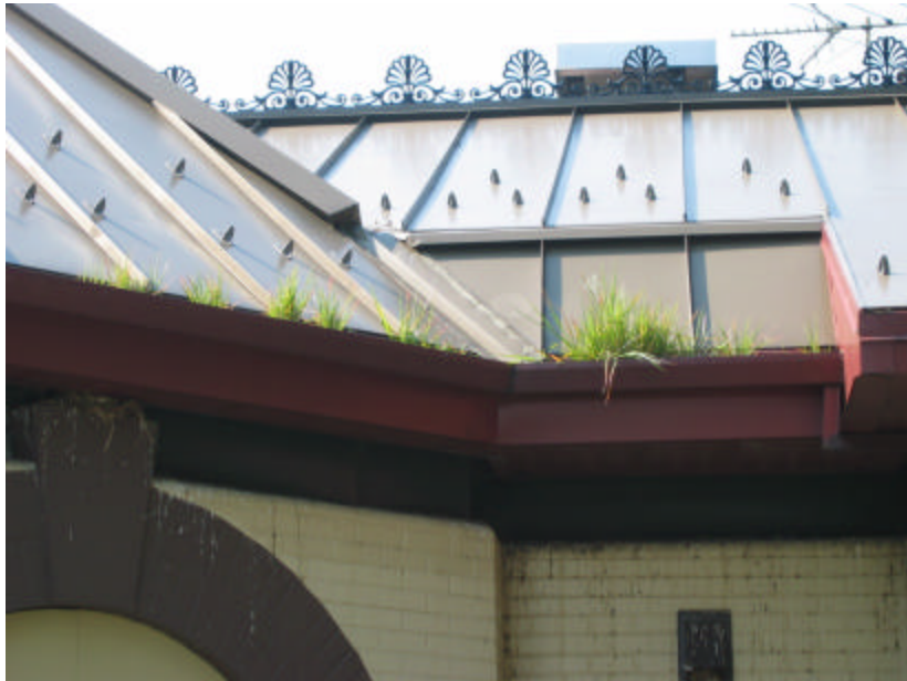
Photo 313 Plants growing in the gutters; note the staining on the bricks.
