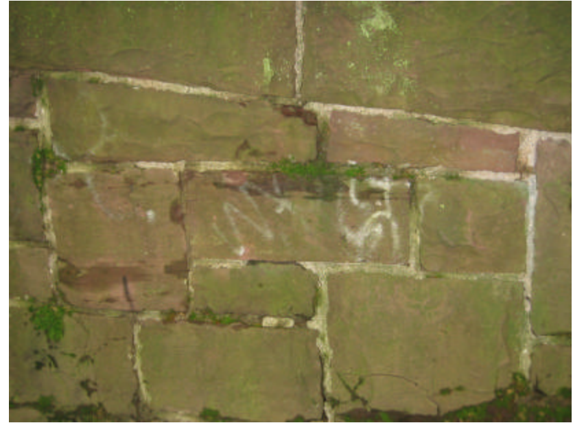
Photo 210 Open and exposed mortar joints on the north cheek wall; note the graffiti and organic growth.
