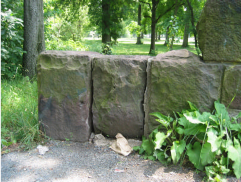
Photo 274 Eroded masonry joints on the east side of the bridge; note that the middle block is displaced and mortar has eroded from its joints.
