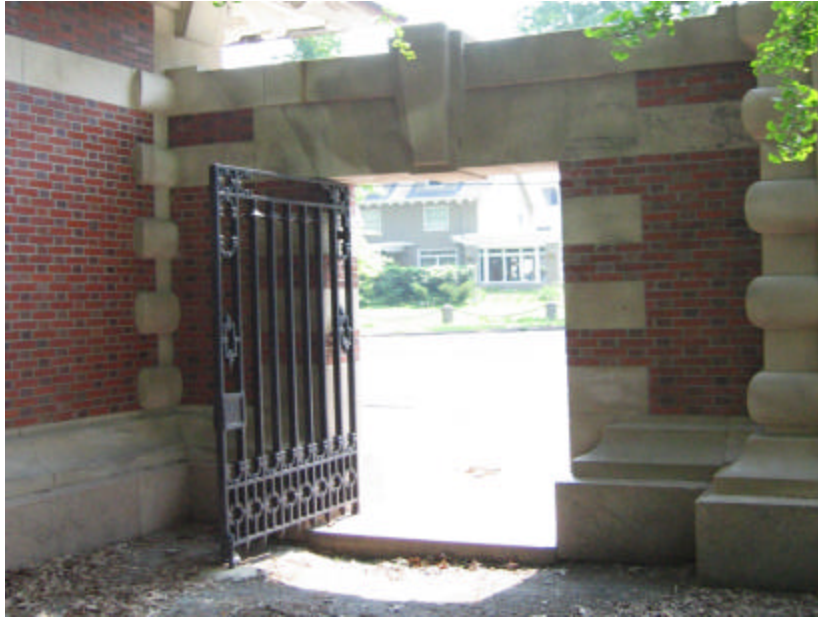
Photo 234 The wrought iron gate in the flat archway adjacent to the north pavilion; note the erosion next to the granite threshold.
