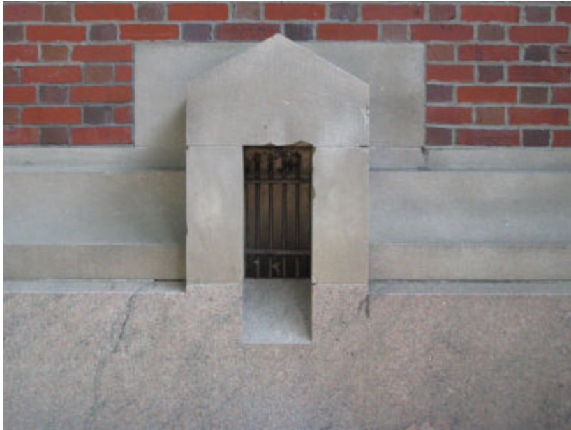
Photo 218 The pedimented limestone vent on the south wall of the north pavilion; note the spalling of the stone.
