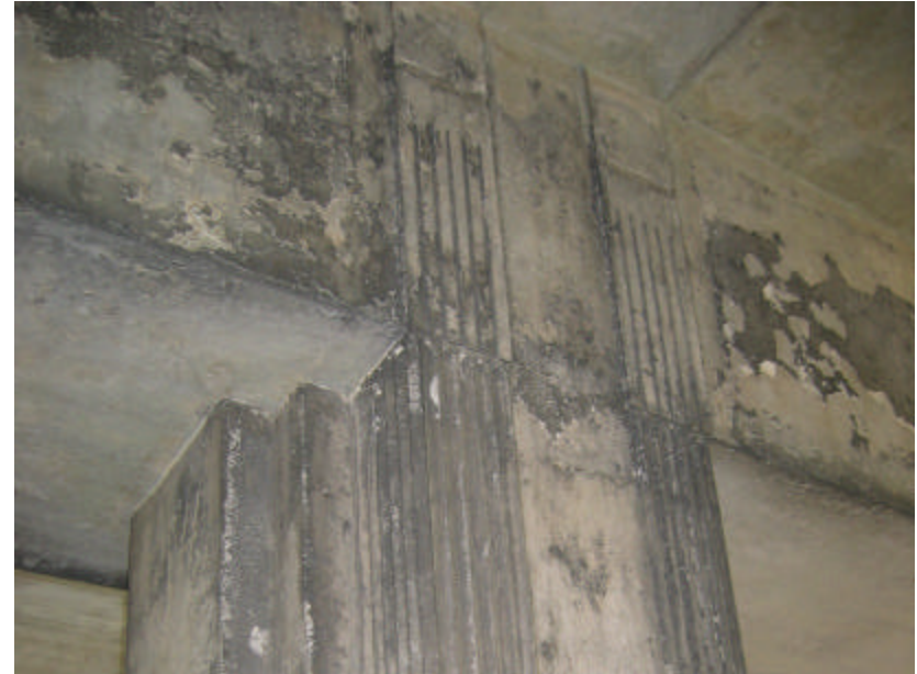
Photo 303 A detail of the concrete surfaces underneath the bridge; note the areas of peeling paint.
