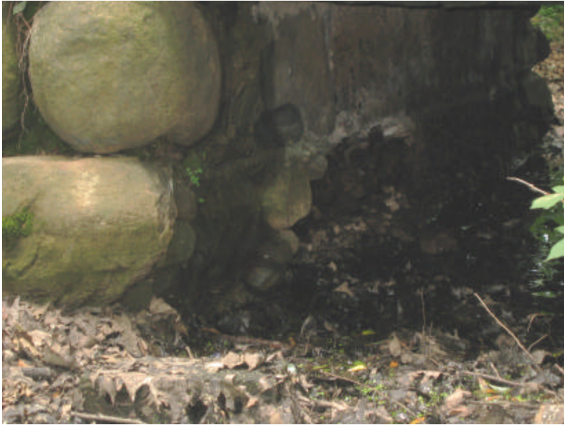
Photo 264 Significant spalling in the concrete box culvert underneath the bridge; note the efflorescence and organic growth.
