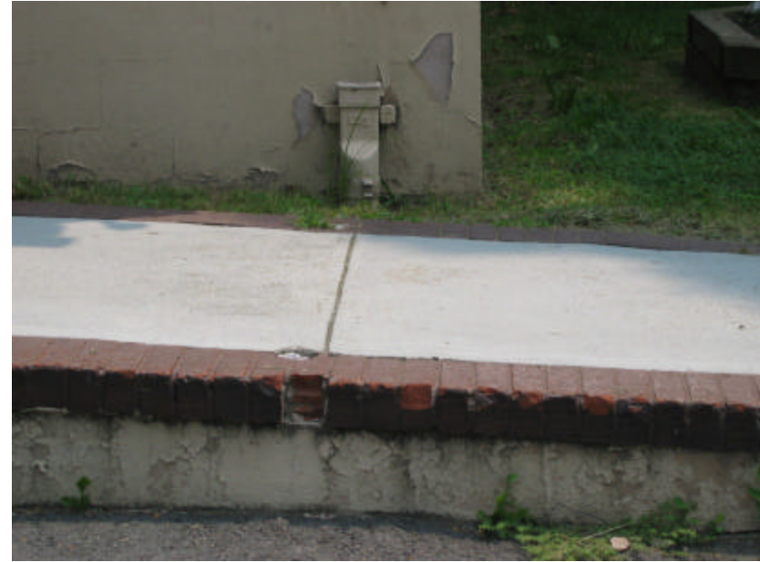
Photo 292 Cracked and chipped brick on the ramp leading to the porch; note the concrete below the brick is stained and soiled.
