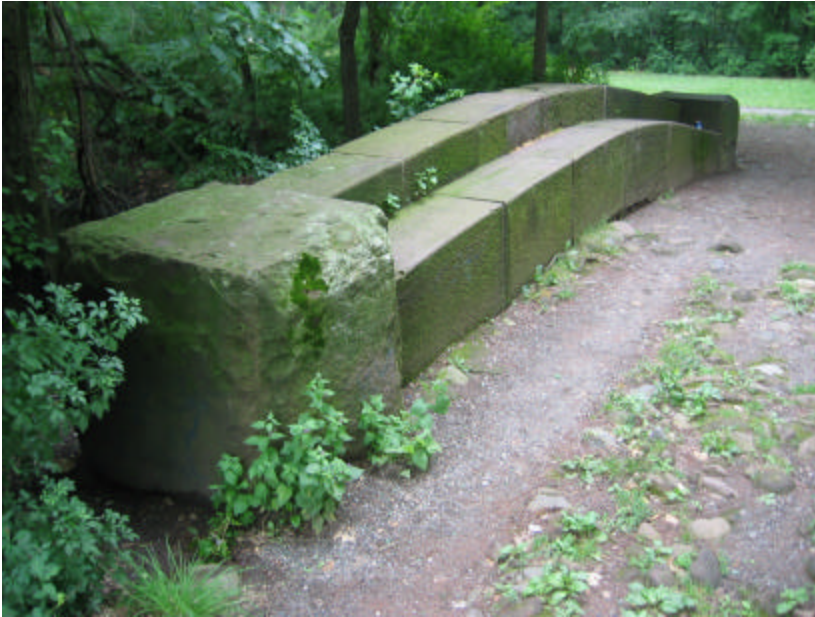
Photo 203 The south bench, copingstones and end blocks of the bridge; note the compacted rock and soil fill that now serves as the bridge's deck, as well as the organic growth at the base of bridge.
