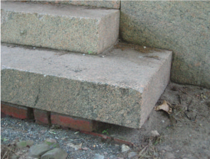
Photo 220 The granite stoop on the west façade of the north pavilion; note the missing brick and the deeply eroded joints.
