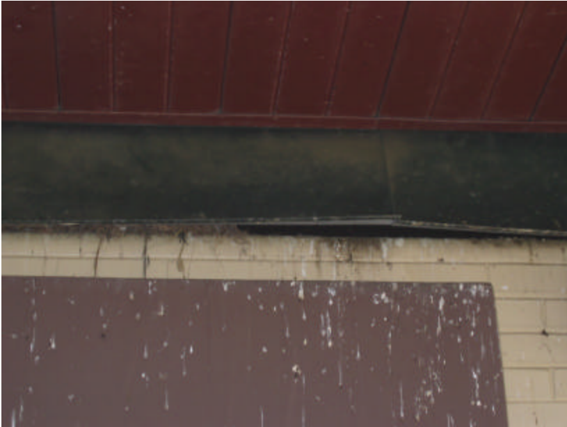
Photo 311 The aluminum cornice on the building's rear has opened; note the bird nests inside and the excrement staining the brick and concrete.
