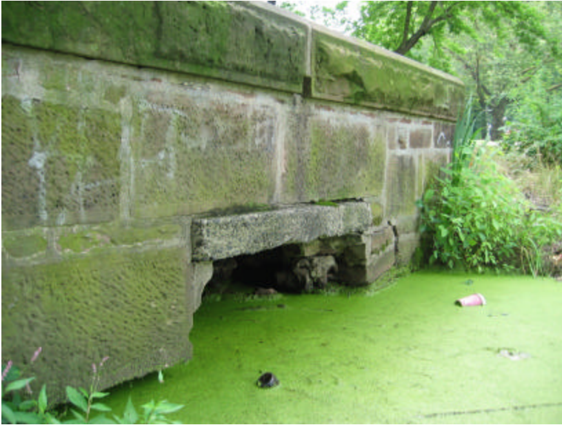
Photo 248 The concrete replacement lintel on the north side of the bridge; organic growth and graffiti; note the limited channel flow area.
