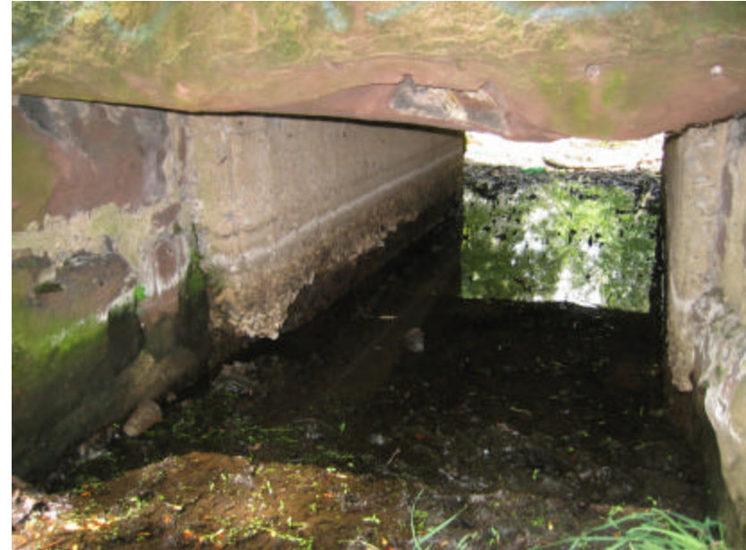
Photo 275 Concrete reinforcing on the bridge's underside; note that the reinforcing has eroded significantly.
