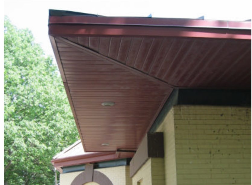
Photo 308 The roof extending over the building; note that it is in good condition.
