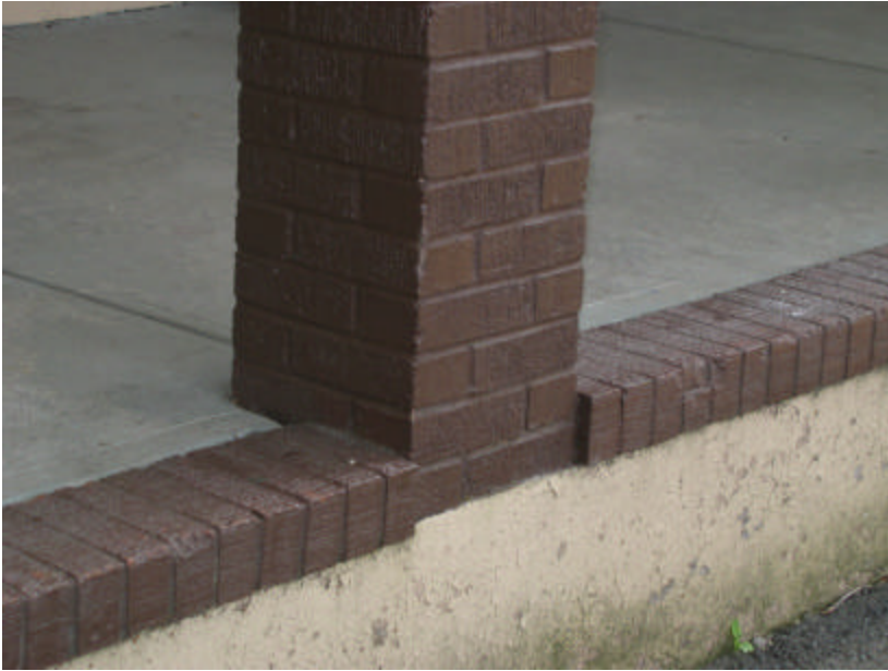
Photo 291 A square brick column and brick trim on the porch; note that the brick is covered with a heavy coat of brown paint.
