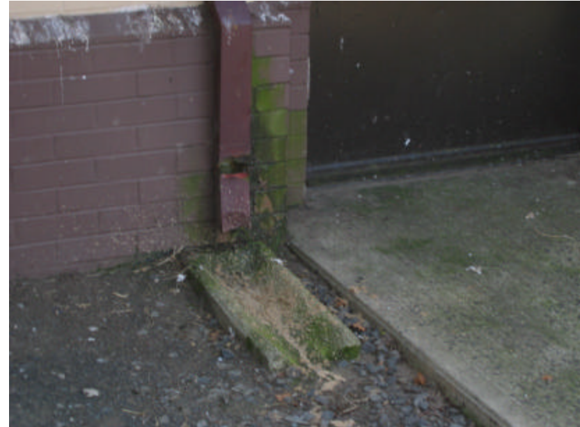
Photo 312 Rusting and damaged downspout; note the organic growth on the bricks.
