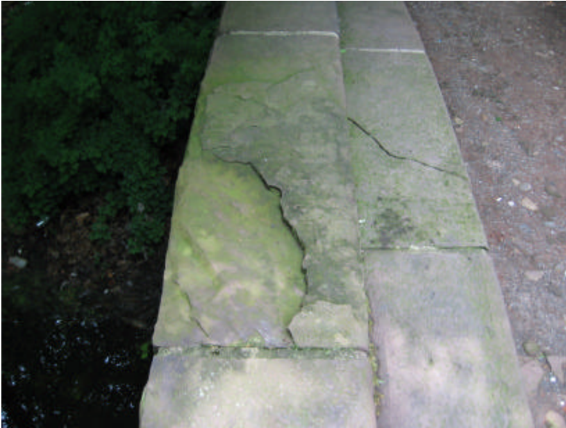
Photo 207 Spalling and delaminating of brownstone on the south copingstones of the bridge; note that cracking and delaminating occurs along the bedding planes of the brownstone.
