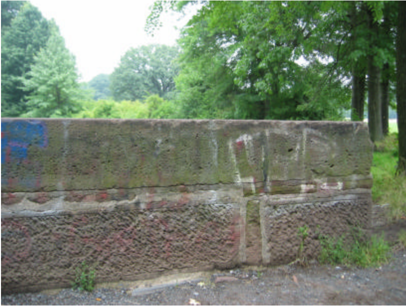
Photo 244 The top course of stone is pock-marked and the vertical tooling has eroded; note the small course of brownstone in the middle.
