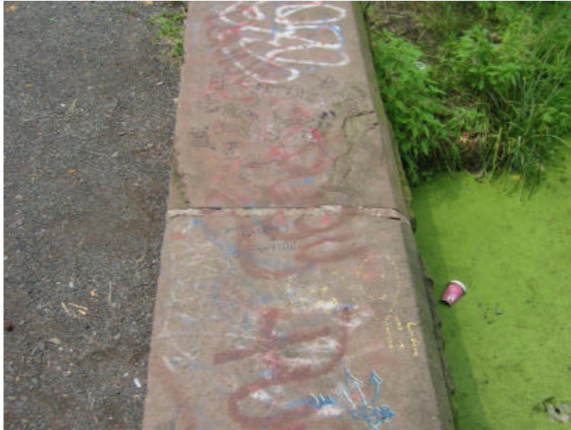
Photo 246 The copingstones atop the north cheek wall; note the spalling and delaminating stone as well as the graffiti.
