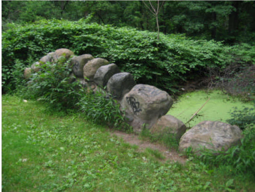
Photo 187 The north cheek wall; note the vegetation and graffiti covering this wall.
