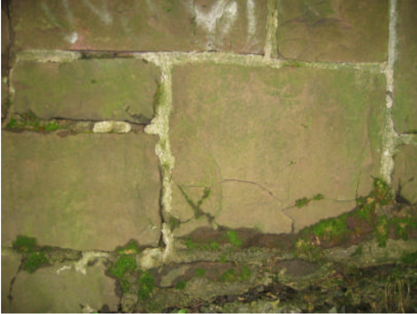
Photo 211 Spalling and cracking stone at the base of the north cheek wall; note the organic growth at the bottom of the photograph.
