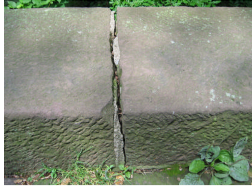
Photo 208 An open and exposed mortar joint between two copingstones at the top of the cheek wall; note the spalling along the edges of the stone and the significant amount of missing mortar.
