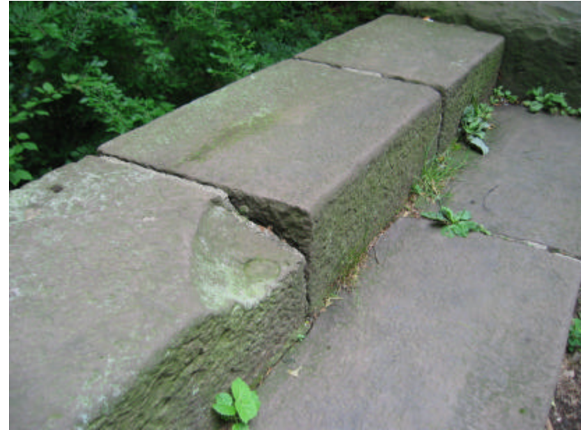
Photo 206 Significant spalling on the corner of a copingstone; note the open and exposed mortar joints with plants growing out of most of them.
