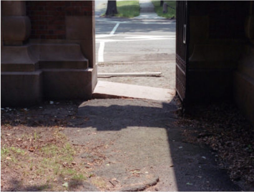
Photo 230 The displaced granite threshold; note the worn-out paving around the site.
