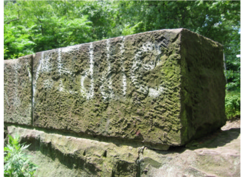
Photo 271 A detail of the brownstone atop the west cheek wall; note that the well-tooled stone surface is spalling and graffiti-covered.
