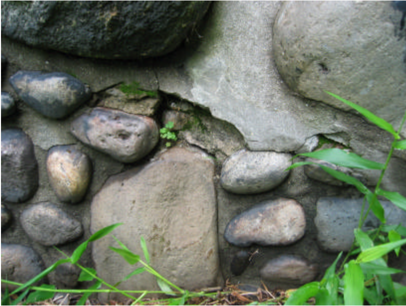
Photo 193 Cracked mortar along the north cheek wall; note the width of the mortar joints.
