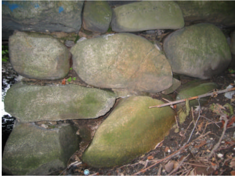
Photo 262 The mortar between these fieldstones on the base of the west cheek wall has eroded significantly or washed away completely.
