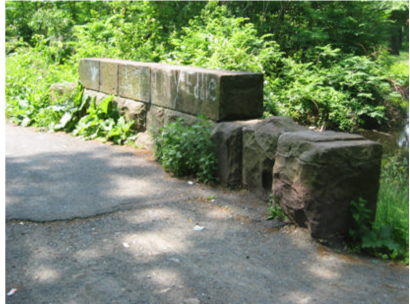
Photo 277 The west cheek wall; note the plant growth at its base and asphalt paving only on the bridge deck.
