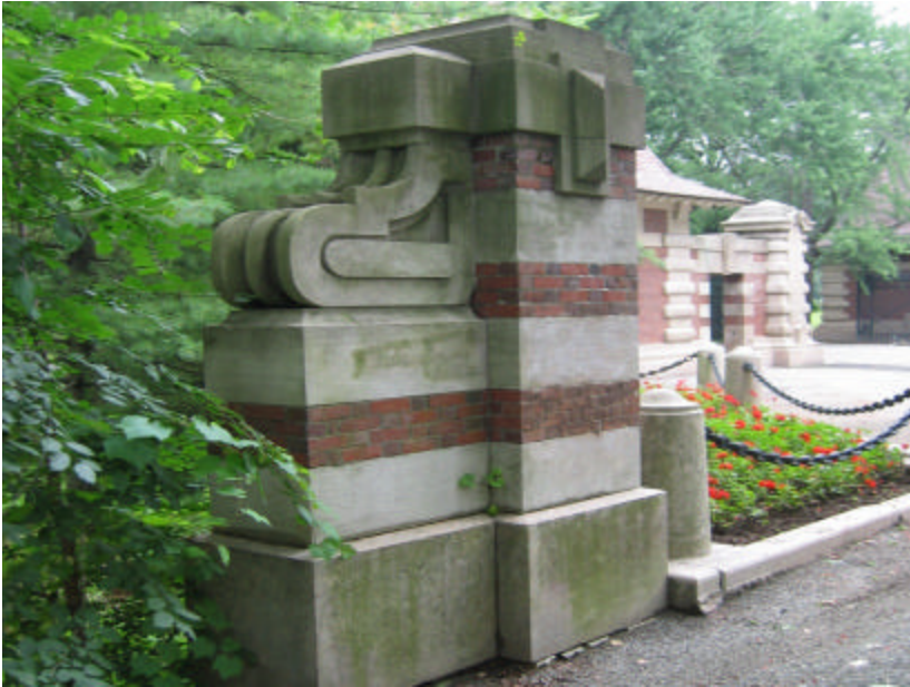
Photo 232 The post at the end of the south fence; note the eroded foundation.
