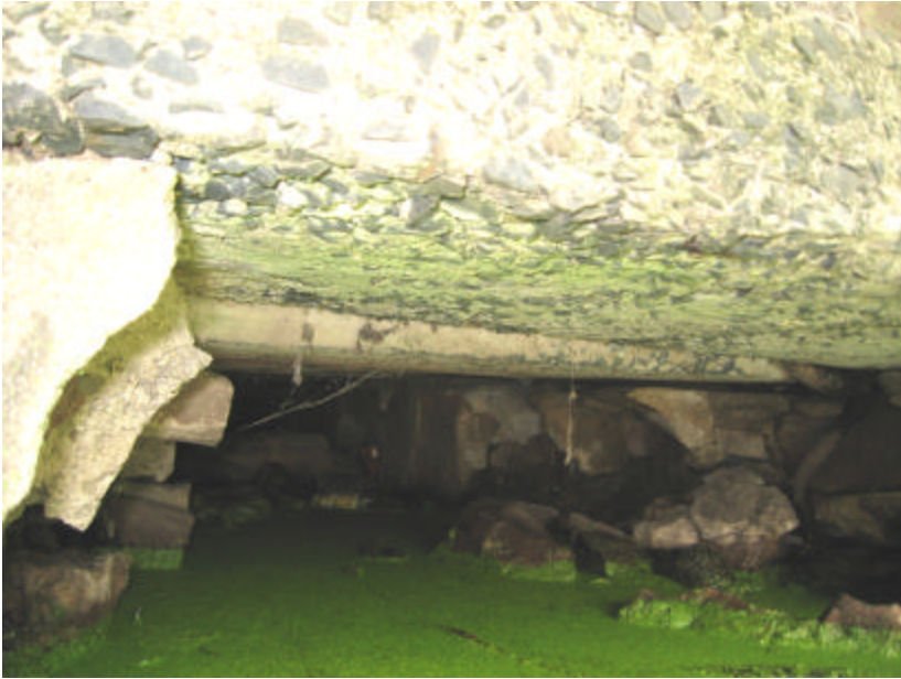
Photo 250 Displaced and broken pieces of concrete and brownstone under the bridge.
