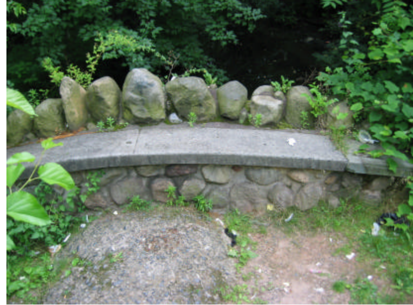
Photo 179 The south bench and copingstones of the bridge; note the plants growing in between the fieldstones and the reconstructed concrete benches.
