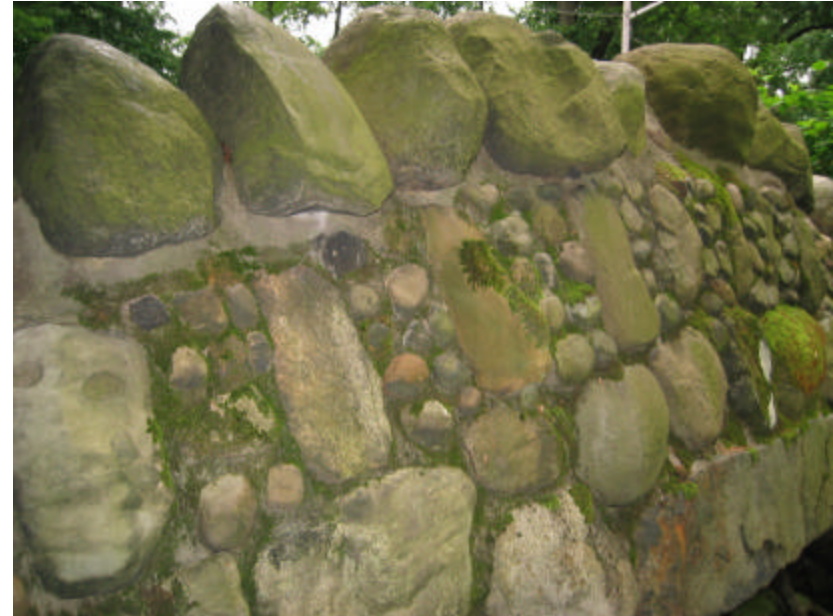
Photo 194 The vertical face of the north cheek wall; note the moss growing on the fieldstone and mortar surfaces.
