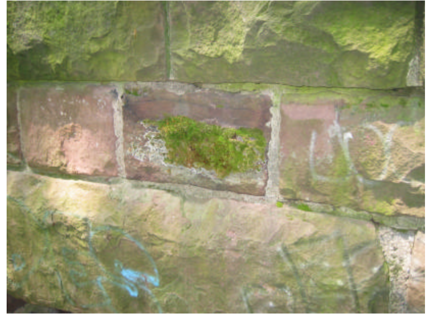
Photo 269 Organic growth and graffiti on the vertical face of the east cheek wall; note the large lintel stone on the bottom of the photo.
