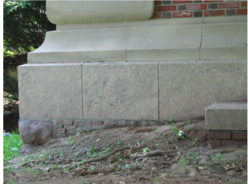
Photo 221 The soil has eroded considerably around the site exposing the foundation.
