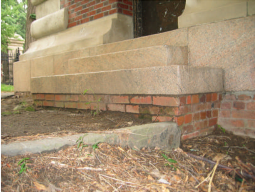
Photo 228 Corbelled brick foundation supporting the stoop; note the erosion around the site.
