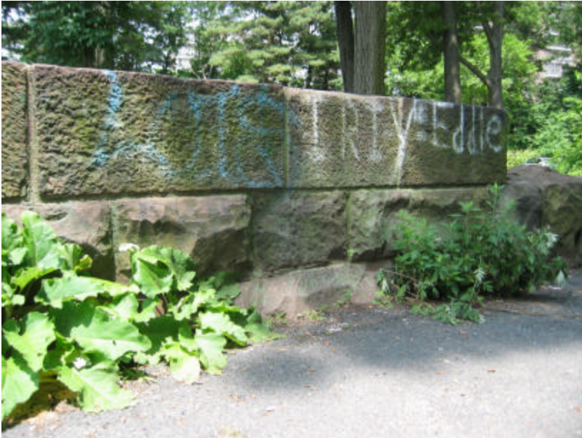
Photo 270 Three courses of stonework on the west cheek wall; note the graffiti on the top blocks and vegetation along the base.
