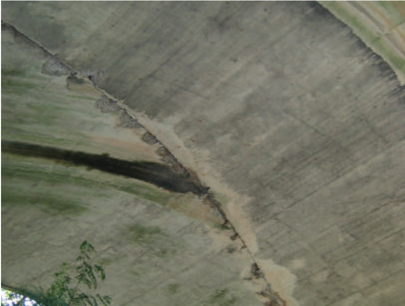
Photo 321 Spalled concrete and water-staining caused by water penetration and the adverse effects of freeze-thaw cycles.
