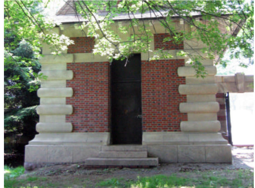
Photo 237 The west façade of the north pavilion; note the original door has been replaced with a sheet of plywood.
