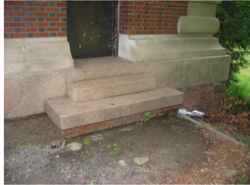
Photo 229 The stoop and doorway of the south pavilion; note the curb extending out from the stoop on the right side of the photo.
