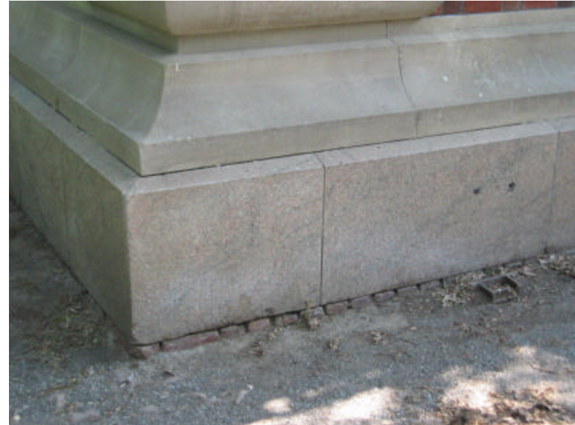
Photo 217 The southwest corner of the north pavilion; note the open and exposed joints of the brick foundation.
