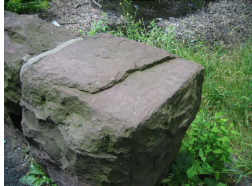
Photo 273 An end block of the west cheek wall; note that the top of this stone has delaminated and the joints have been repointed.
