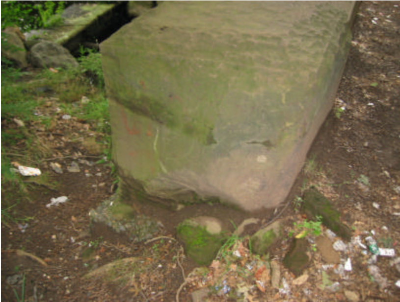
Photo 199 One of the large brownstone blocks at the west end of the north cheek Wall; note the exposed concrete foundation, and the rocks and roots suggesting significant water runoff causing erosion.
