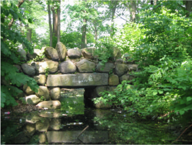
Photo 260 A large granite lintel spanning the culvert opening on the bridge's west side; note the change in the water level from the photo below.
