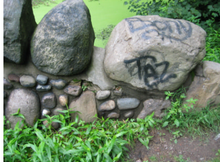
Photo 192 Visible signs of graffiti, erosion and spalled, cracked mortar on the north cheek wall.
