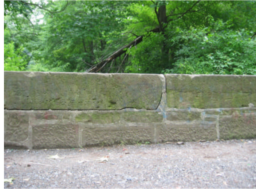
Photo 245 The cracked bed joint at the base of a copingstone on the south cheek wall.
