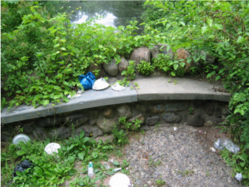
Photo 182 The north side of the bridge and built-in bench; note the vegetation and garbage covering the path and bench.
