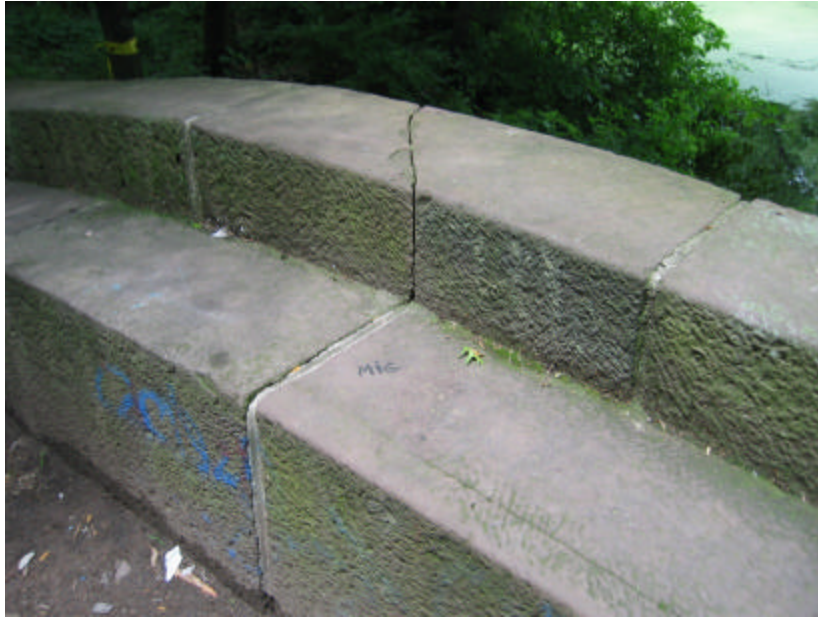
Photo 205 This copingstone is cracked in half; note how the crack matches up with the open and exposed mortar joint on the bench, suggesting that cracking may have been exacerbated by water infiltration and freeze-thaw cycles.
