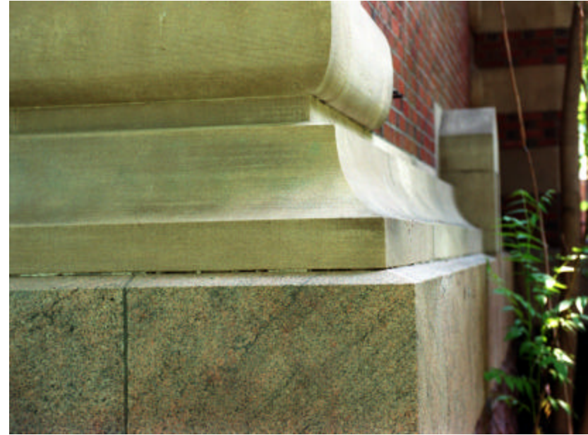
Photo 227 The southwest corner of the south pavilion; note the open and exposed vertical and bed joints.
