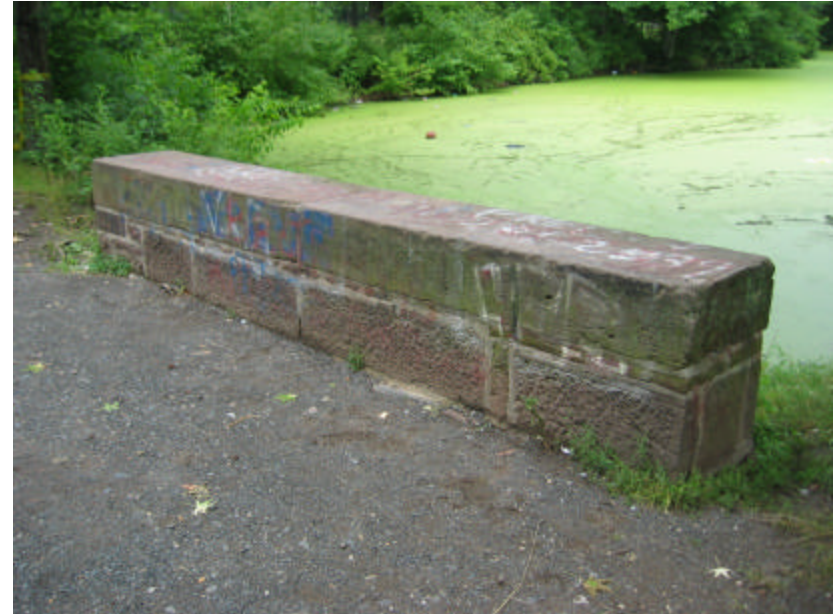
Photo 241 View of the north cheek wall; note that the surface is covered with graffiti and organic growth.
