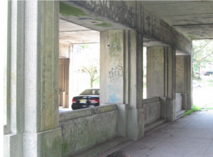
Photo 295 Four columns and a low wall that support the concrete slab over which the train tracks run.
