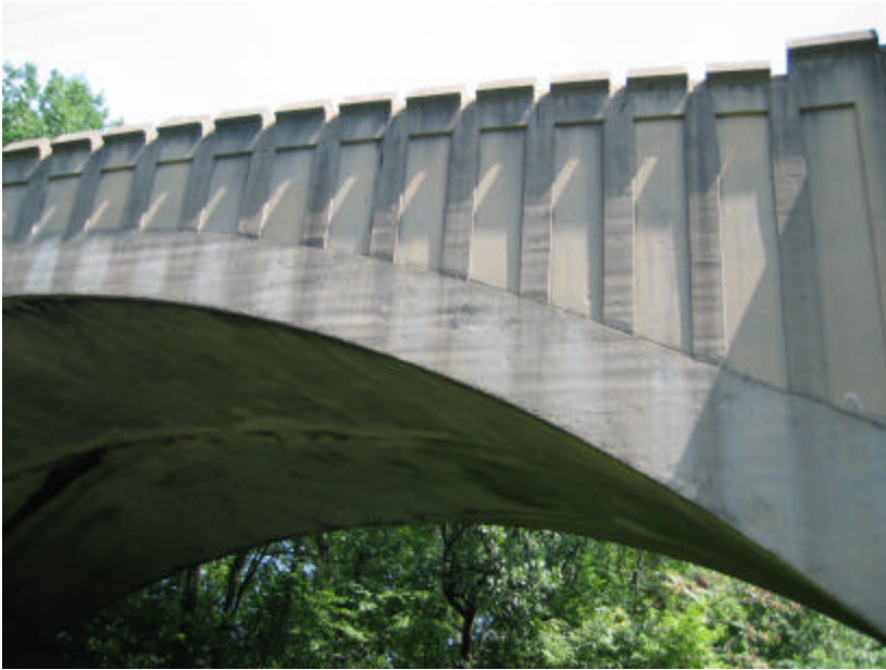
Photo 319 Spalling is visible at the base of many vertical sections; note the crenellated parapet wall.
