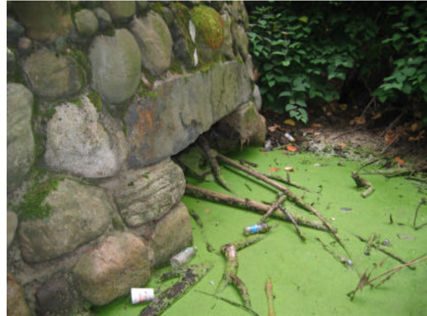
Photo 190 Debris and sedimentation clogging the culvert on the north side; note the organic growth covering the fieldstones and mortar joints.
