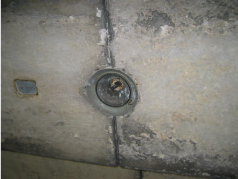
Photo 304 One of the broken recessed lighting fixtures on the underside of the bridge.
