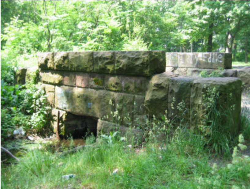
Photo 276 The coursed-ashlar and rough-cut brownstone, east cheek wall; note the green organic growth and spalling stone surface.
