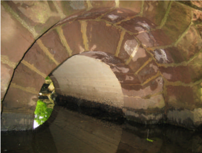
Photo 201 The two brownstone arches on the south side of the bridge; note the efflorescence and water staining of the brownstone blocks.
