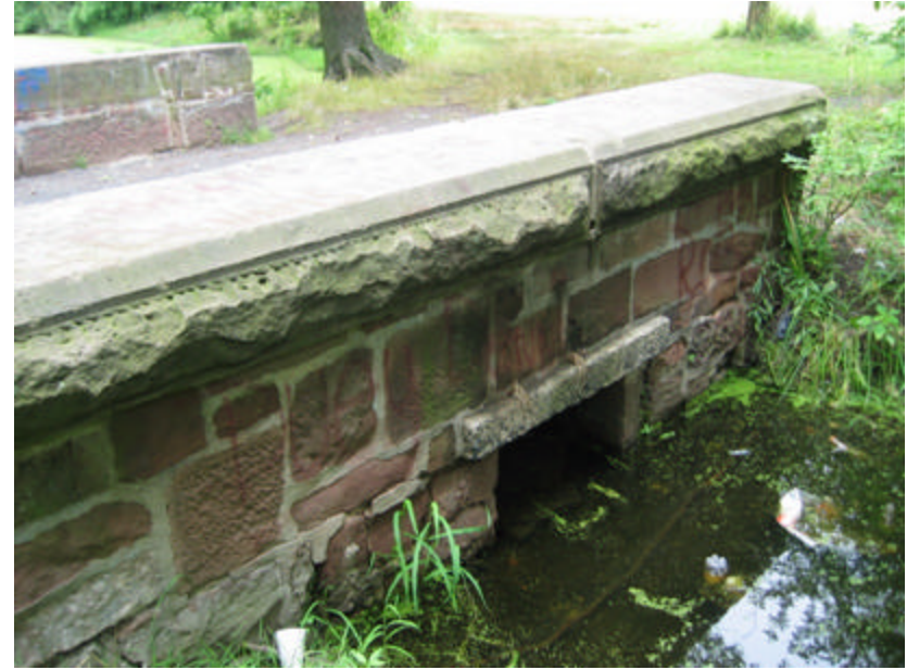
Photo 247 Missing and eroded mortar and brownstone at the base of the south cheek wall; note the dressed, beveled edges and rough-cut surfaces on the copingstones. Note also the limited water flow area of the channel opening.
