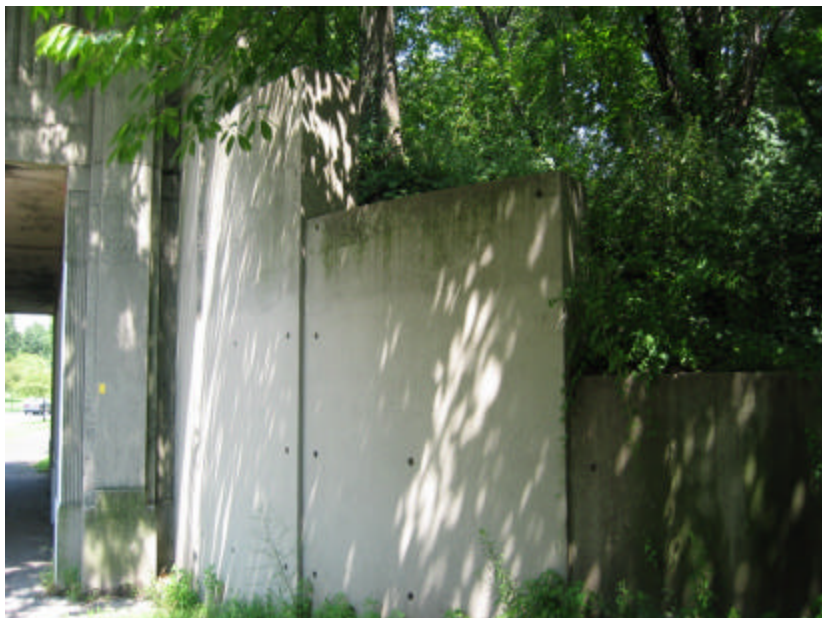
Photo 296 One of the stepped wing walls arching out away from the bridge; note that a section of the wall is painted.
