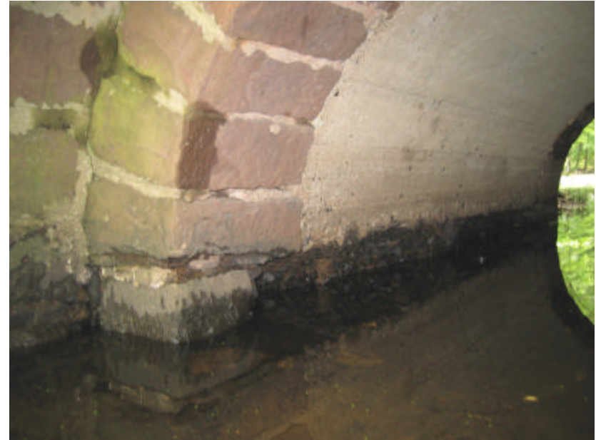
Photo 202 The brownstone arches and concrete archway under the bridge; note the significant erosion of the brownstone blocks, mortar joints and the concrete arch.
