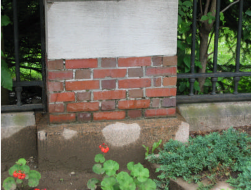
Photo 224 Open and exposed mortar joints at the base of a post; note that there are open vertical joints at the granite base.
