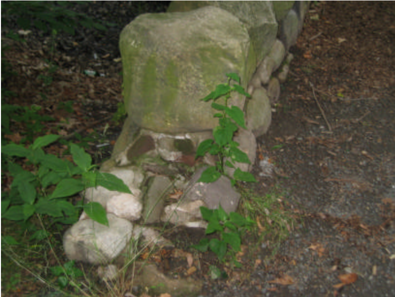
Photo 266 Fieldstones missing from the south side of the west cheek wall.
