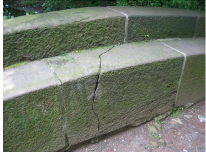
Photo 204 This large crack, approximately 3/8" wide, goes entirely through the brownstone block; note the eroded mortar joints, brownstone and soil at the base of the block.
