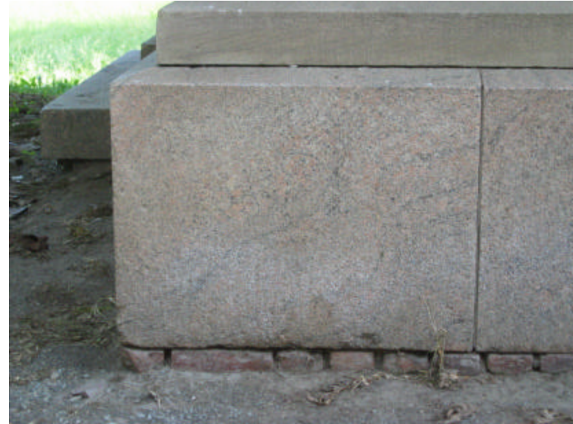
Photo 219 Granite plinth resting on the brick foundation; note the open vertical and bed joints of the granite and limestone.
