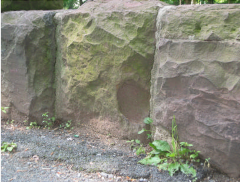
Photo 272 An area of circular spalling on the middle block; note that the top fifth of the block on the right has been reattached or replaced with new brownstone.
