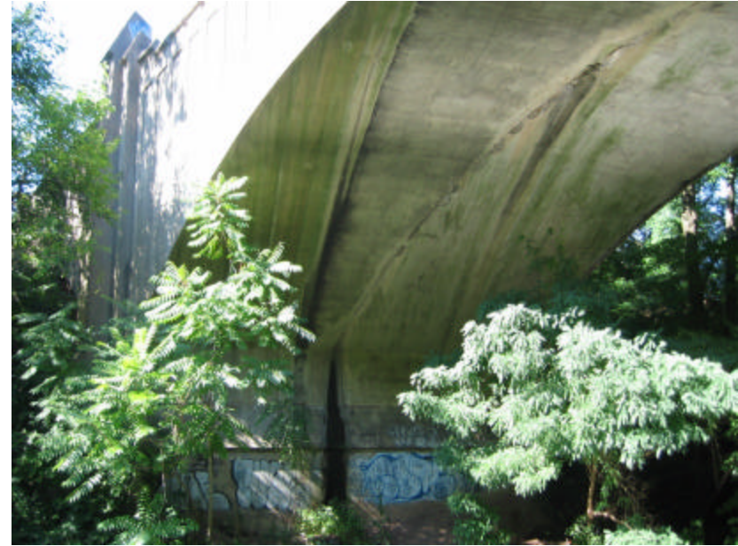
Photo 320 Black staining caused by water damage is visible on the arched span as well as on the foundation caps; note the graffiti and other types of soiling.
