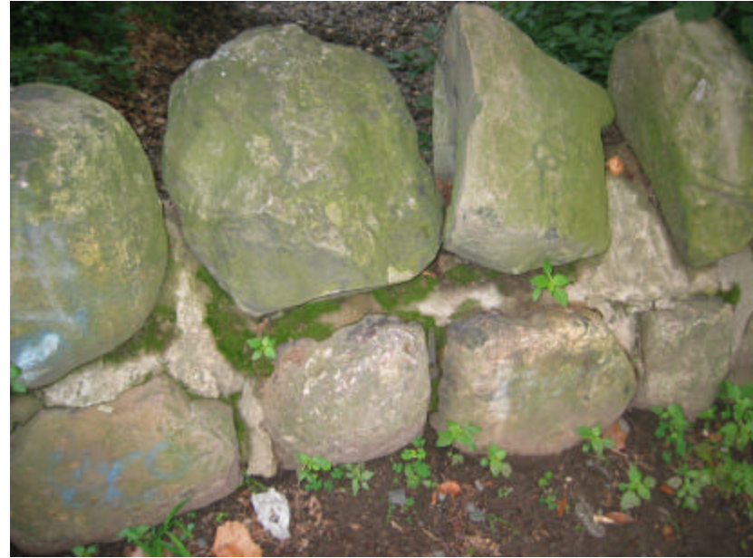
Photo 259 The bottom course of stonework on the bridge capped by large fieldstones; note the wide mortar joints and the moss on the wall.
