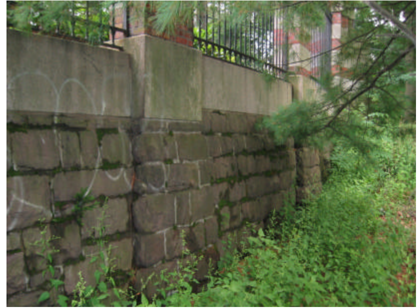
Photo 233 The brownstone retaining wall of the south pavilion; note the moss and graffiti covering the mortar joints and brownstone.
