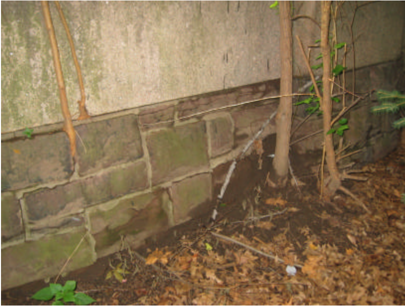
Photo 226 The brownstone retaining wall extending from the north pavilion; note that trees are growing out of cracks in the wall.
