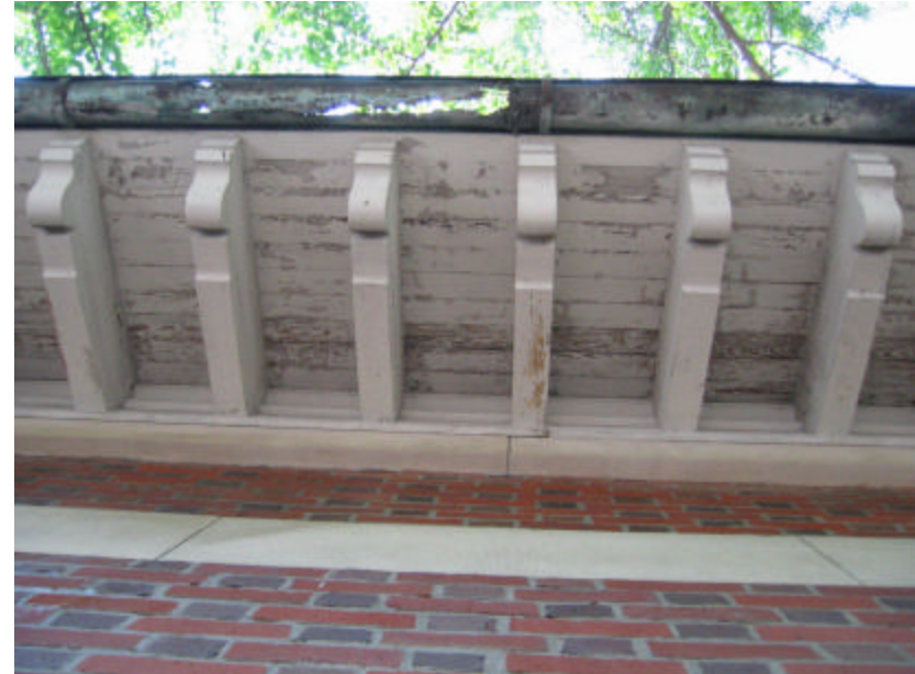
Photo 239 Completely corroded gutter on the north pavilion.
