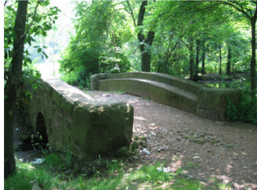
Photo 198 View looking east over the Brownstone Bench Bridge; note the rough and uneven condition of the bridge's deck.
