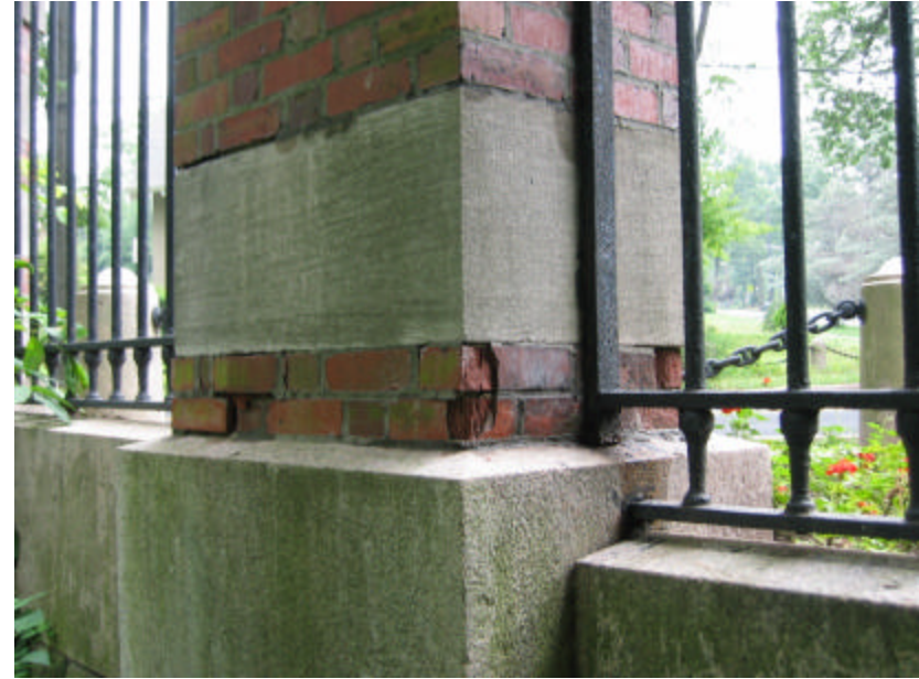
Photo 225 Spalled and cracked brick at the base of a post; note the poor condition of the bed joints between the limestone and brick.
