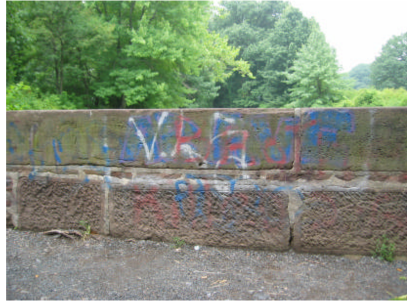
Photo 243 The courses of brownstone on the north cheek wall; note the different finishes on the stone surfaces as well as the graffiti.
