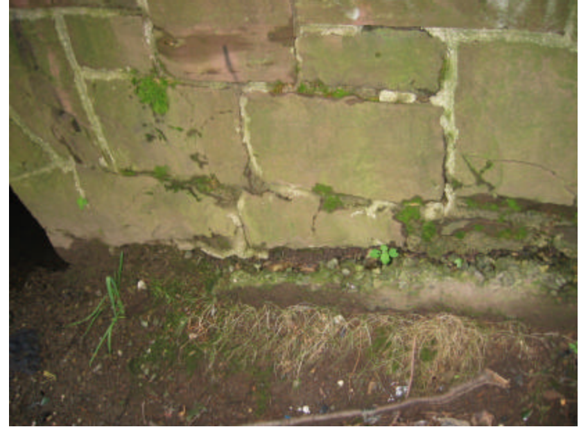
Photo 212 Cracked and eroded concrete foundation at the base of the north cheek wall.
