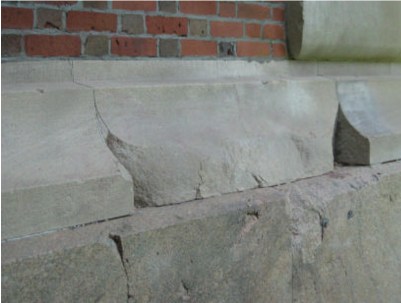
Photo 222 Severe spalling and cracking of the limestone and granite base on the north pavilion.
