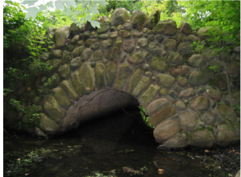
Photo 183 The vertical face of the south cheek wall; note the rustic fieldstone design of the bridge and concrete arch.
