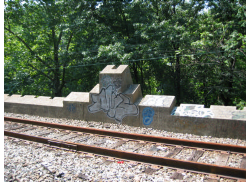
Photo 318 The parapet wall and pier cap on the west side of the bridge; note that large sections of the concrete surfaces are covered with graffiti.
