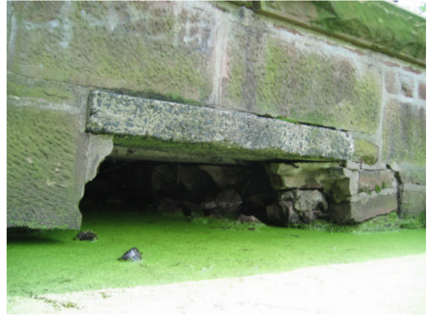
Photo 249 Cracked and missing brownstone and mortar on both sides of the bridge.
