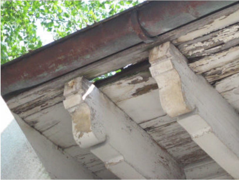
Photo 236 Severely rotted beaded wood board sheathing on the north pavilion.
